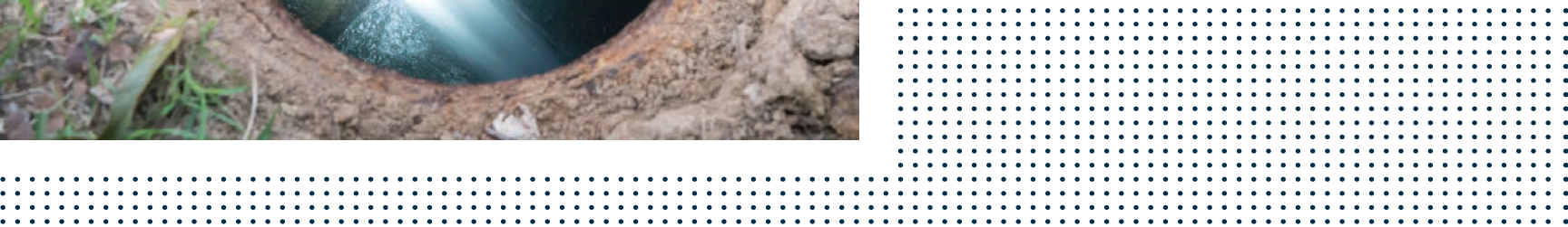
<< Water flows back into a manhole while Chris Hooker (out of frame) jets a sewer line.
